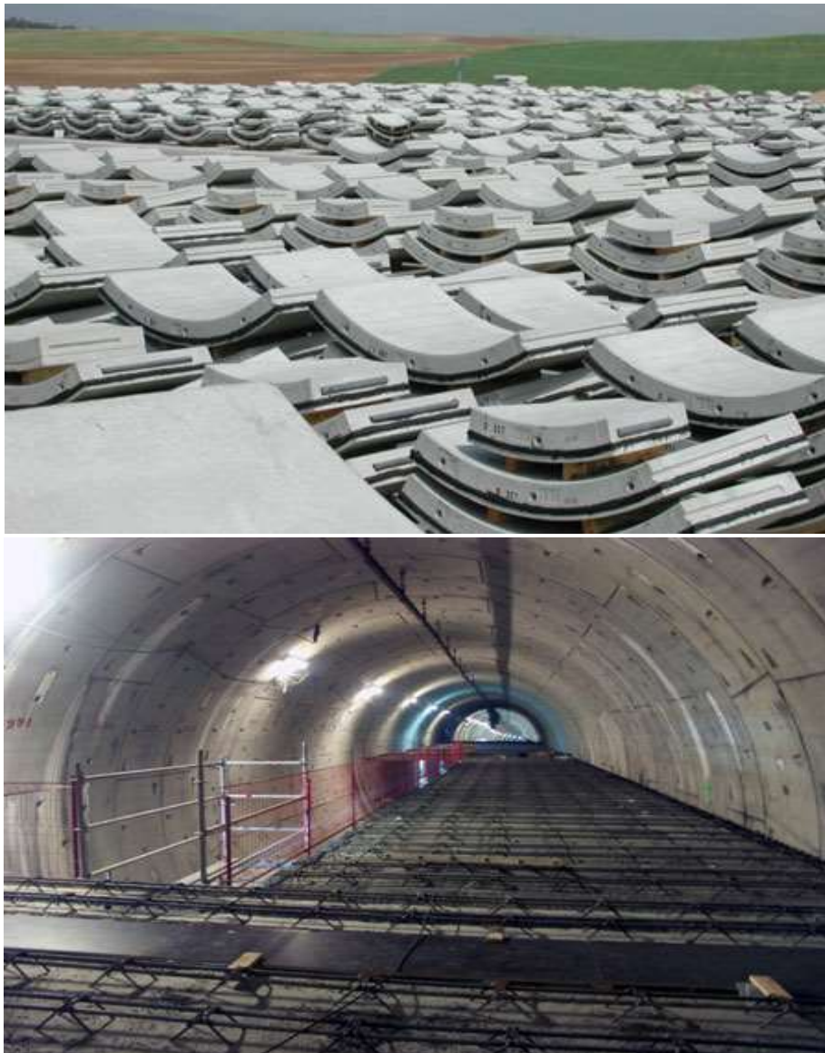
Image 3-20. Circular tunnel with voussoirs and voussoir manufacturing plant.
